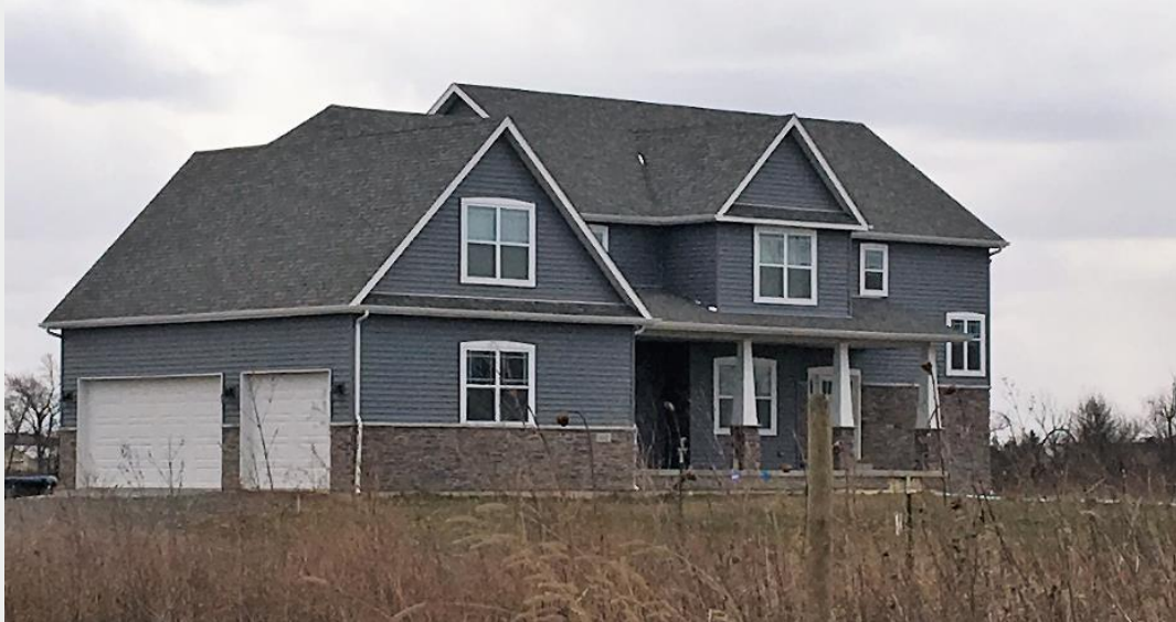
4,255 square foot estate home under construction, adjacent to Portage Solar Farm (Solar Farm 6) On-site pond, pool and attached garage (cost estimated at $465,000) April 2018
